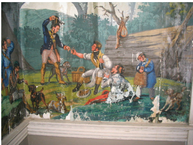
Fig. 6. This water-damaged panel with flaking paint surface was adhered to an exterior wall to the left of the front door
