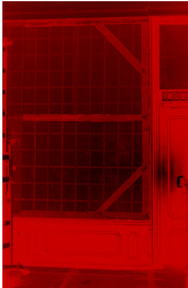
Fig. 1 Boards of plywood and lattice frames, both fitted within the original battens, cross members and corner braces.
